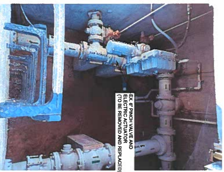
PHOTO 6 - PALMER AVE. TANK VALVE VULT
