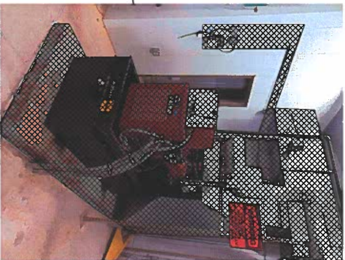
PHOTO 10 - PALMER AVE. TANK EXISTING GENERATOR
